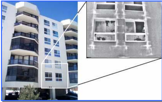
Thermal image of water leakage around windows.
